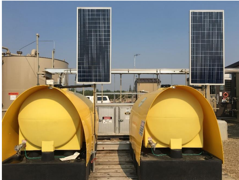
Figure 2-2 Project pumps (solar pumps)
