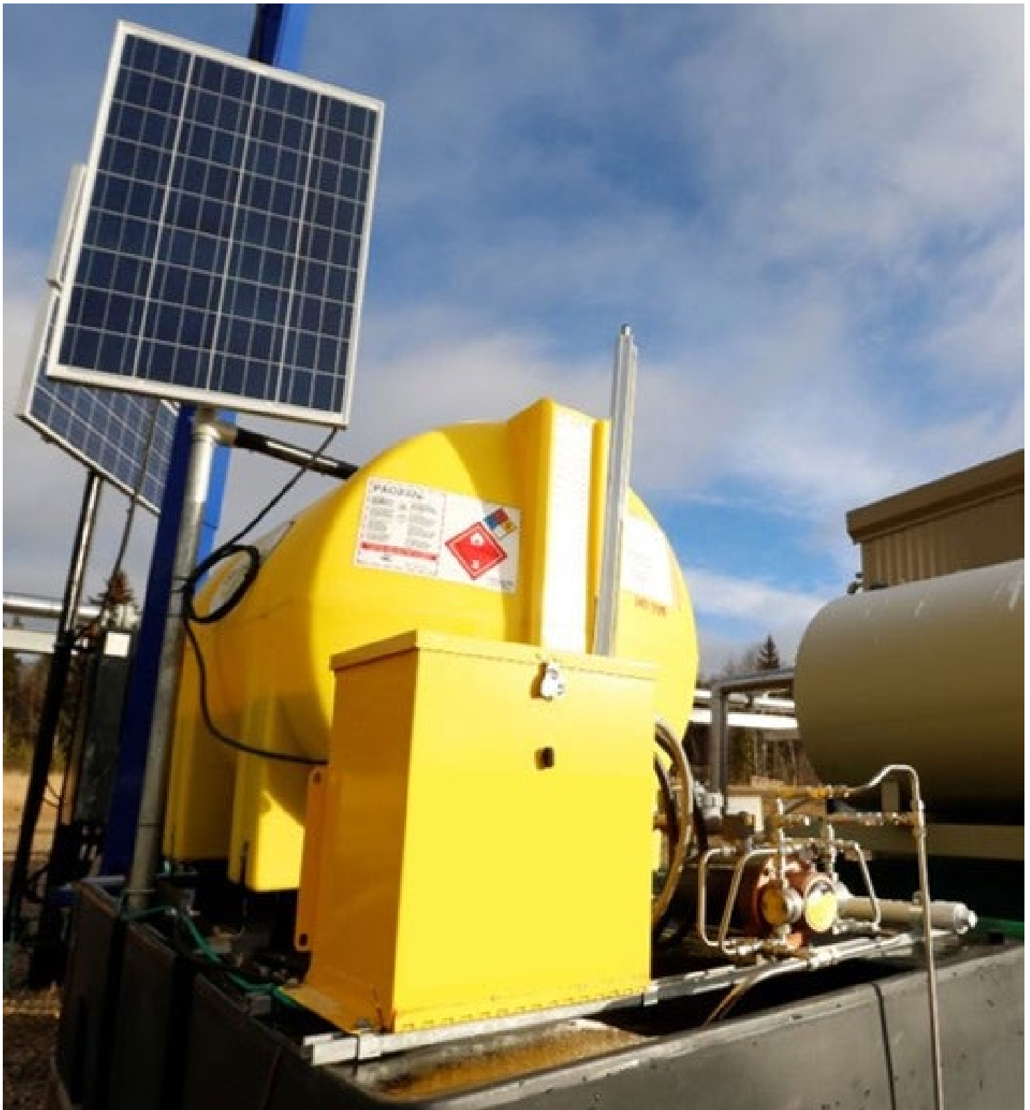
A solar-powered pump that replaced a natural-gas operated and methane venting pneumatic pump.
