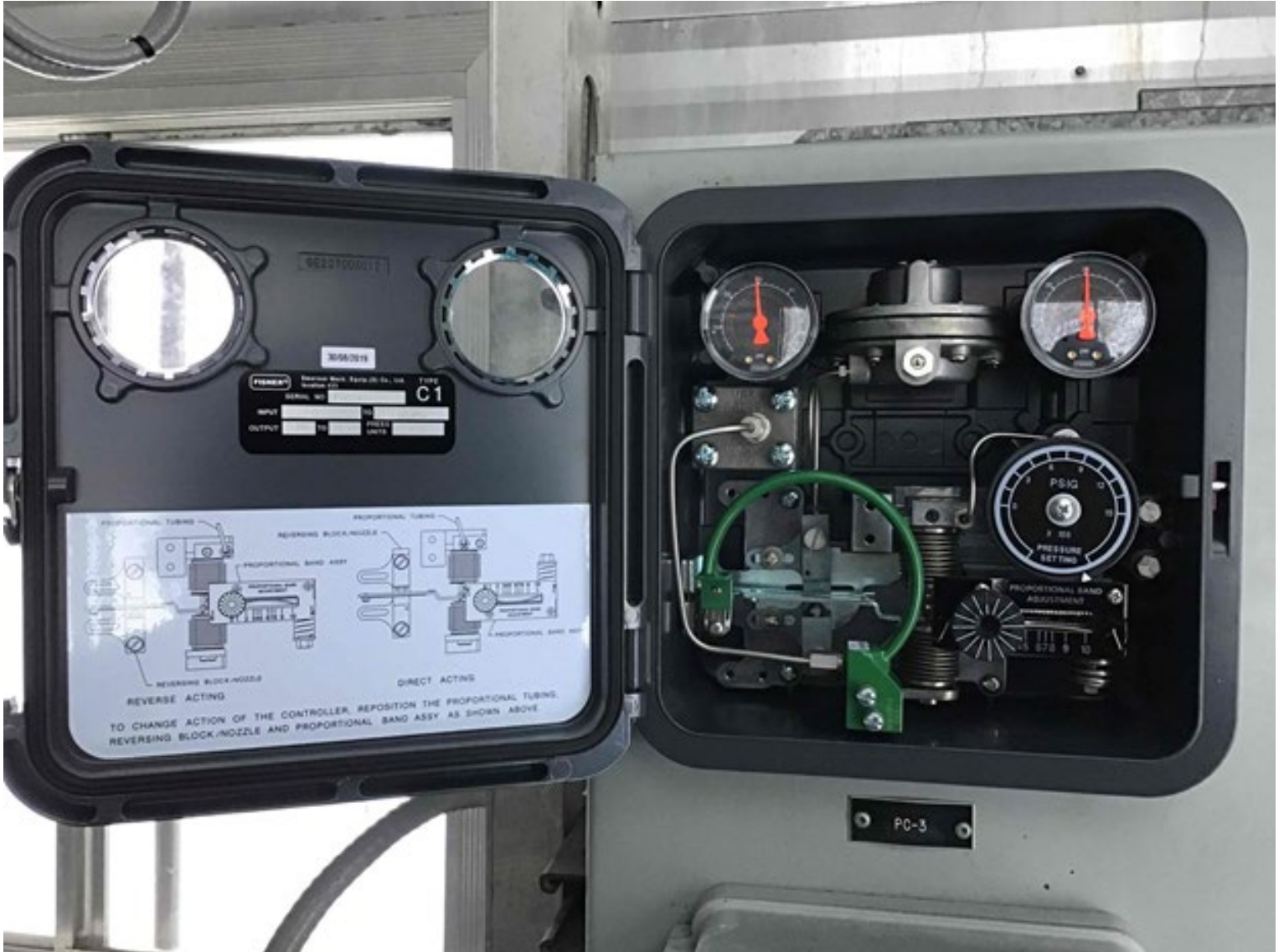
An example of an instrument that was converted to leak less methane into the atmosphere.
